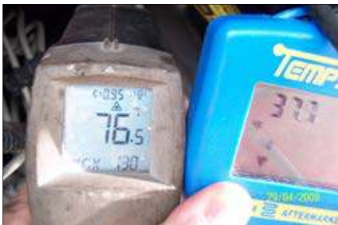
Figure 7: This is a typical reading that can be expected when taking temperature readings on an A/C system with an infrared temperature gun. Both the infrared gun on the left and the contact type temperature reading tool on the right are reading the temperature on the same metal suction line about 1/2-inch apart. Before doing the test, I felt the suction line with my hand, and it felt like a glass of iced tea. The reading on the contact type temperature reading tool indicates a temperature that would be expected of a glass of iced tea. However, the infrared gun indicates a temperature that is almost 40° higher. This was despite numerous efforts to get an accurate reading with it and was the lowest temperature recorded.
